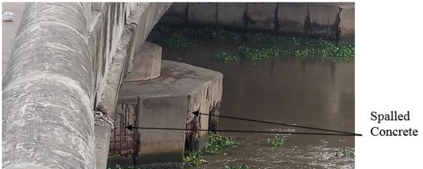
Figure 1: Concrete spalling of the pile cap of Carter bridge in Lagos, Nigeria.
