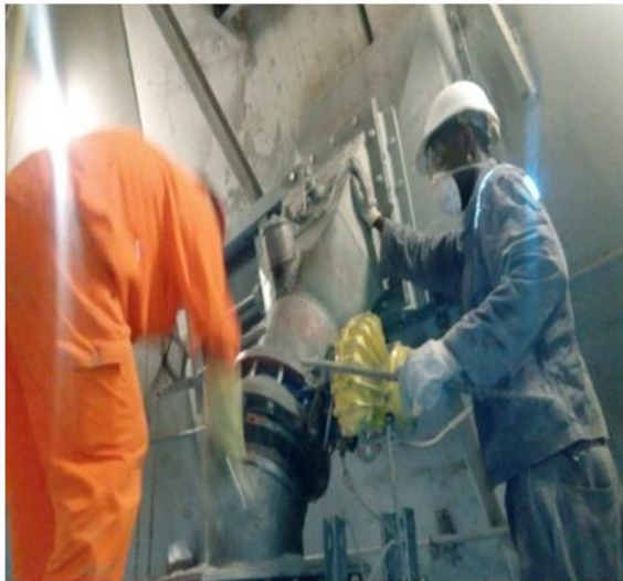
Figure 9: Cement silo (caked cement) cleaning
