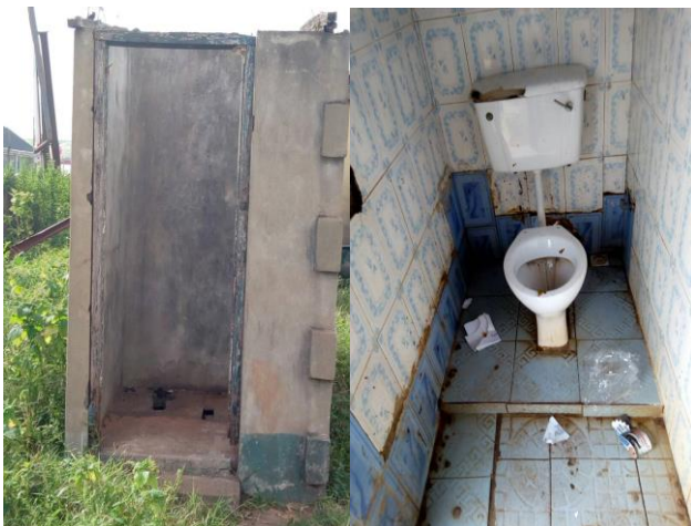
Figure 4: Dilapidated sanitary facilities
